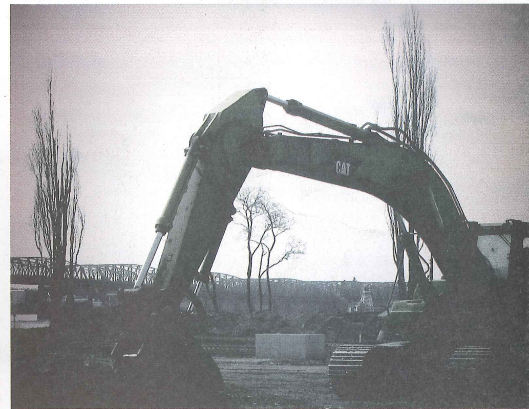
Excavation has begun, and the first buildings are slated to open mid-2017.
