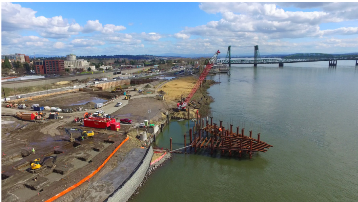
A photo taken by an aerial drone shows the progress at The Waterfront Vancouver. Falseworks at the site of the Grant Street Pier are visible in the river, and straw covers a park area in the background.
