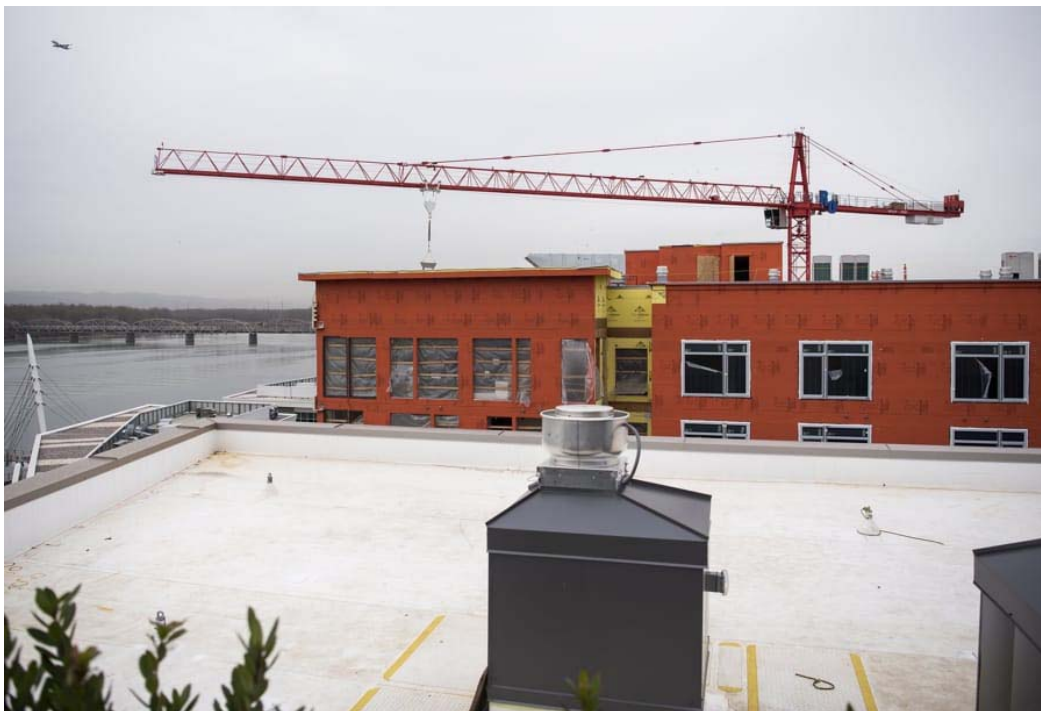
The crane for the Riverwest apartment building came in below the height limit, but it sits very close to the roof of the finished structure. Alisha Jucevic/The Columbian
