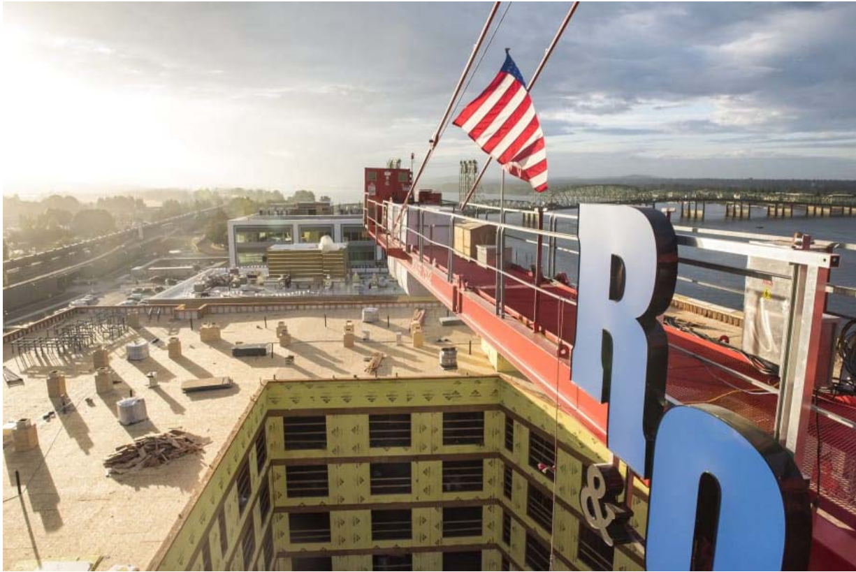
A R&O Construction tower crane operated in September, helping to build The Murdock and Rediviva buildings at The Waterfront Vancouver. Pearson Field is located just past the treeline on the left. Nathan Howard/The Columbian
